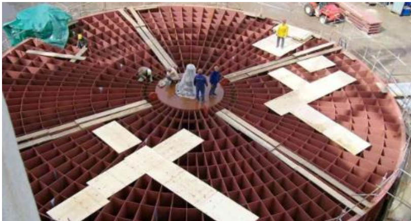
21m-diameter air preheater for Walsum, Germany
