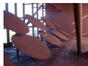
Static mixers inside ESP's inlet assembly stage
